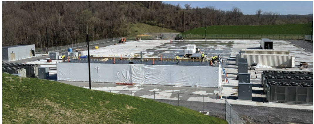
Site work is underway at the West Virginia High Technology Consortium campus in Fairmont for a new NOAA supercomputer.
